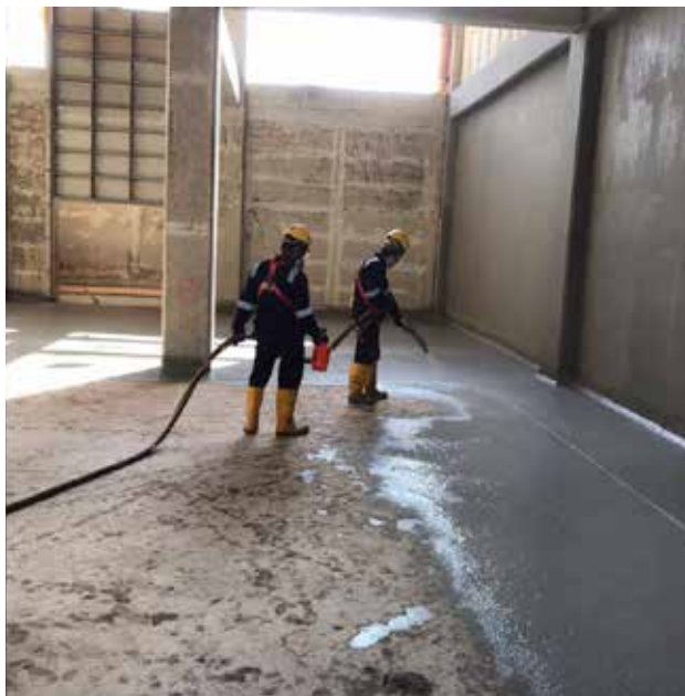
Rapid refinery Pengerang, Malaysia: Tank refurbishment with Sikalastic®-1K (spray application), Sikadur® Combiflex® SG Tapes and Sikaflex® PRO-3.
