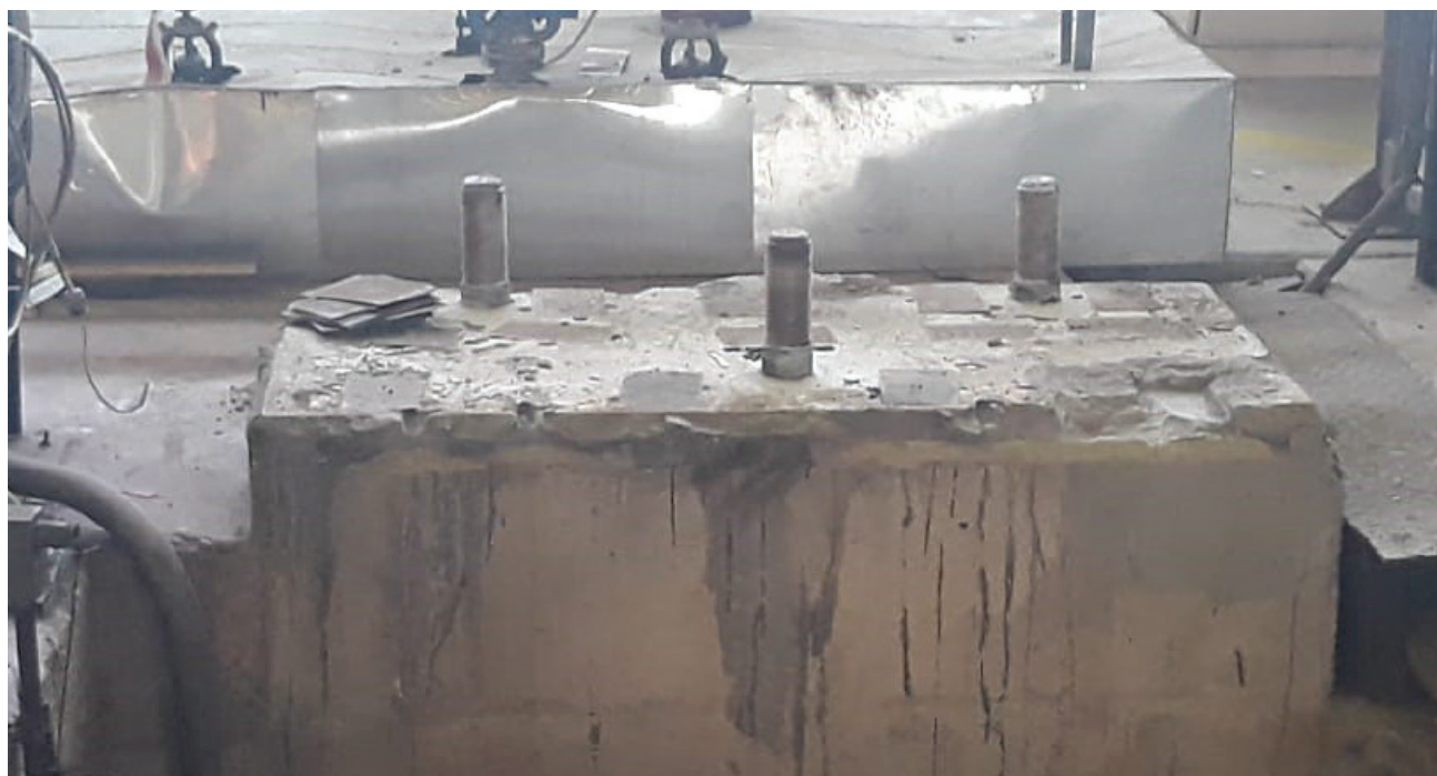
Concrete base with cracks, displacement problems and deformations.
